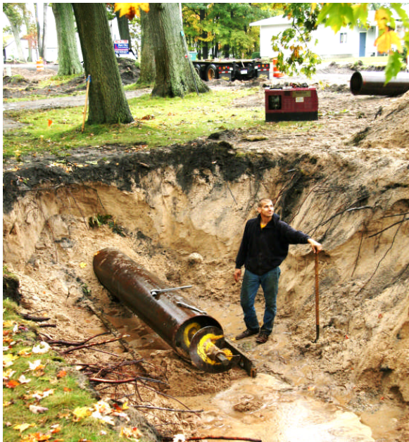
To the left is a photo of the "jack and bore" process used to save as many trees as possible within the construction route.
